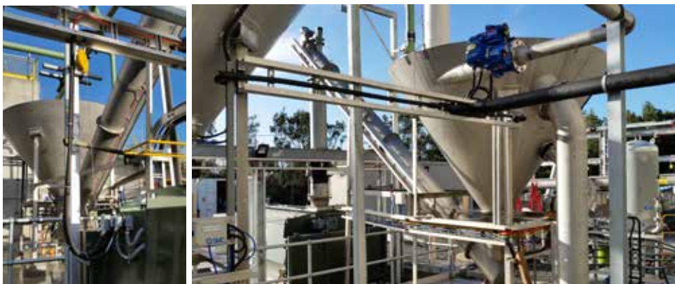
SANDWASH™ and SPIROTAINER®: Grit washing and storing
