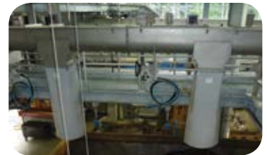
Truck outloading system
